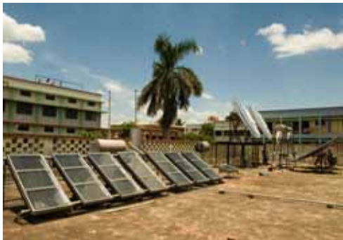
Solar systems on the roof at Tripolia Hospital, Patna
